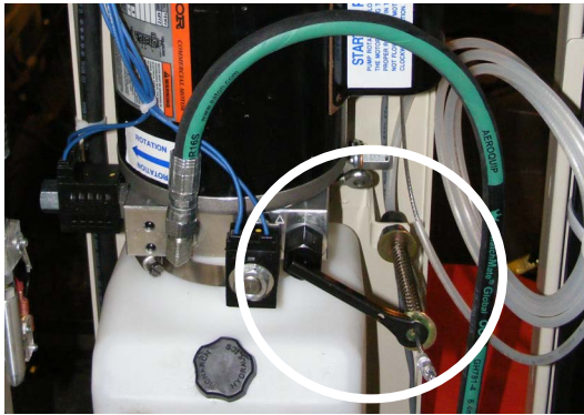
Figure 22 Manual lowering lever and cable in tower
